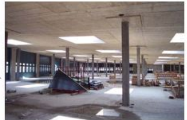
Inside Phase 1 Primary System
