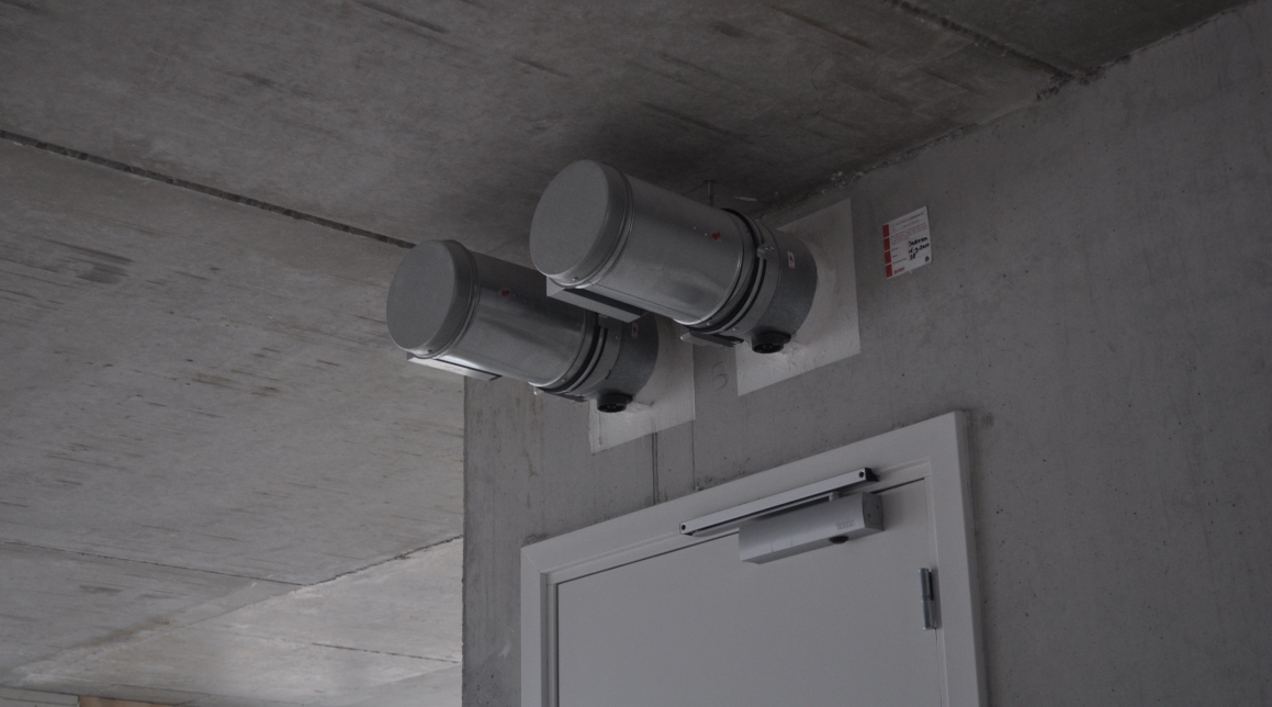
Base building air handling connections
