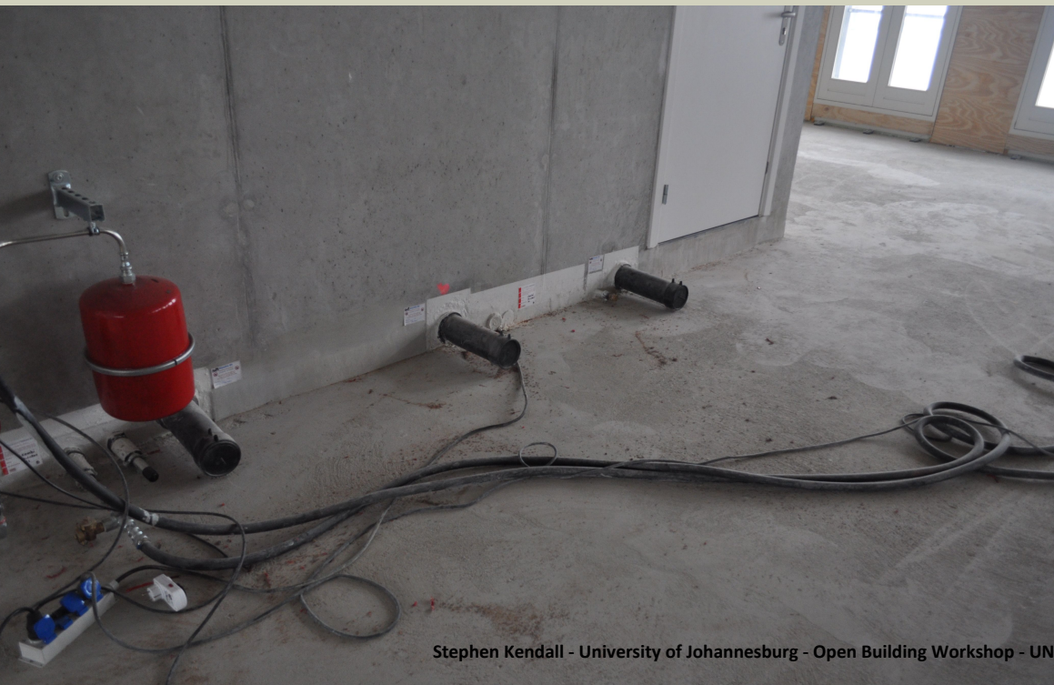
Base building drainage pipe connections (the tenant floor is 15cm lower than the corridor floor)
