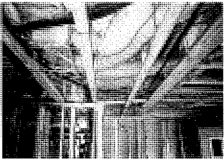
The entangled service systems in the floor cavity of a normal residential project, 1993.
