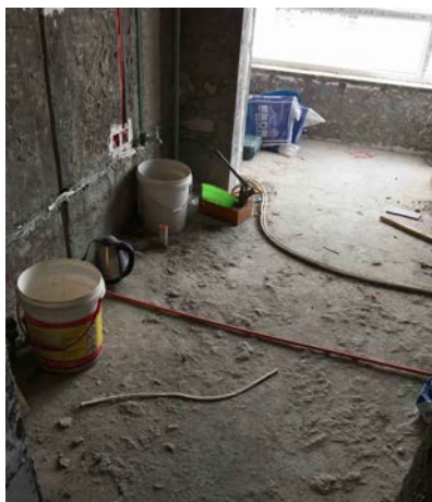
Gas piping and meter/ Shower drain from upper floor
