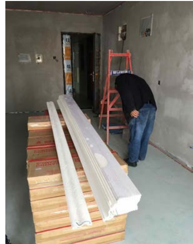
To conceal new wiring at the top of the walls, plaster "cove" molding will be installed (the white products)
