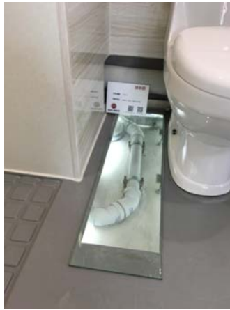
WC is rear discharge; drain pipe under floor is from the shower
