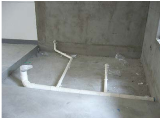
Depressed floor at the bathroom only
