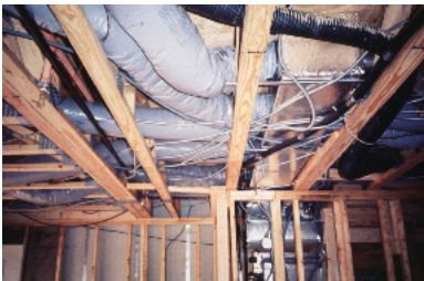
Fig.1 The entangled service systems in the floor cavity of a normal residential project, 1993.
