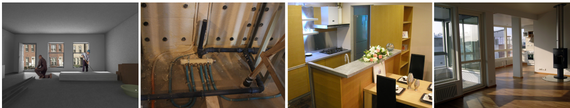
IMAGE 10-13: Multi-skilled installers at work; fit-out piping installation; finished dwellings ready for occupancy one month after the fit-out work began.
