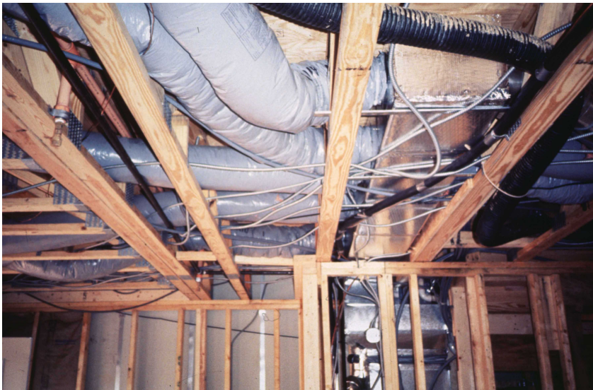
Figure 1: Entangled wiring and piping in a typical US dwelling
